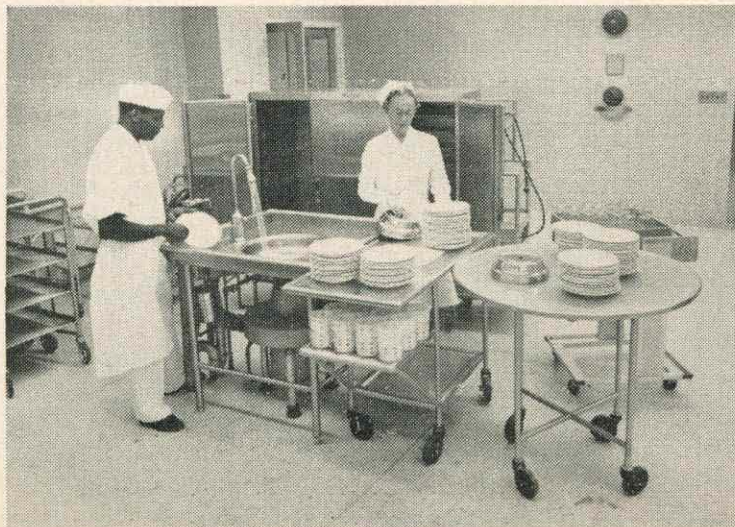
A unique feature of the rehabilitation hospital's kitchen equipment is the dishwashing area. In the left photo, Claydean Lewis and Miss Jean Alexander, assistant director of dietary services, prepare the dishes for the flight washing machine. The breakdown equipment shown here consists of a waste disposal unit, a small, rectangular mobile table and a circular, rotating stacking
