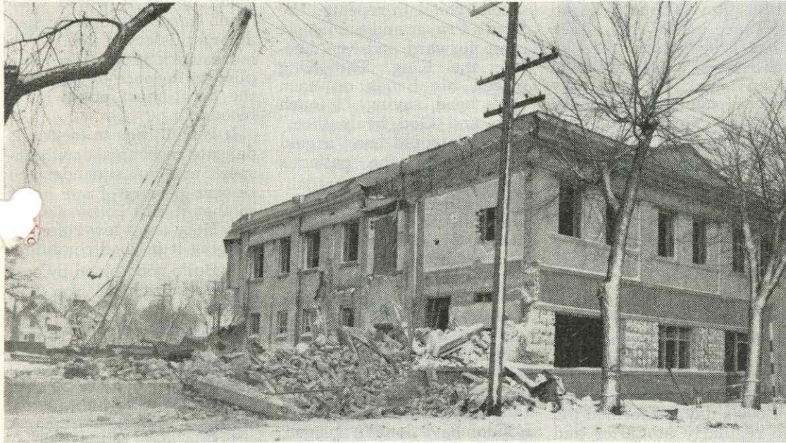
The old Central Tuberculosis Clinic on Winnipeg's Bannatyne avenue went down under the wrecking machinery of R. Litz and Sons this month to pave the way for the construction of The Manitoba Rehabilitation Hospital. Tenders for the Sanatorium Board's new, six-storey hospital will be called April 18, and construction will begin at the end of May. (Photo by David Portigal & Company.)
